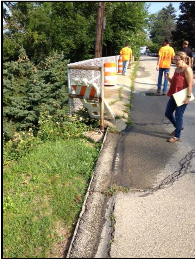
Photo of Cantilever Walkway on Kaufmann Avenue (notice, existing fencing and railing. No guiderail.)
